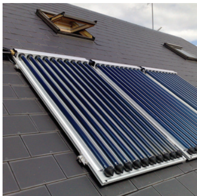
Evacuated Tube collectors
