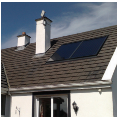
Flat Plate in-roof collectors
